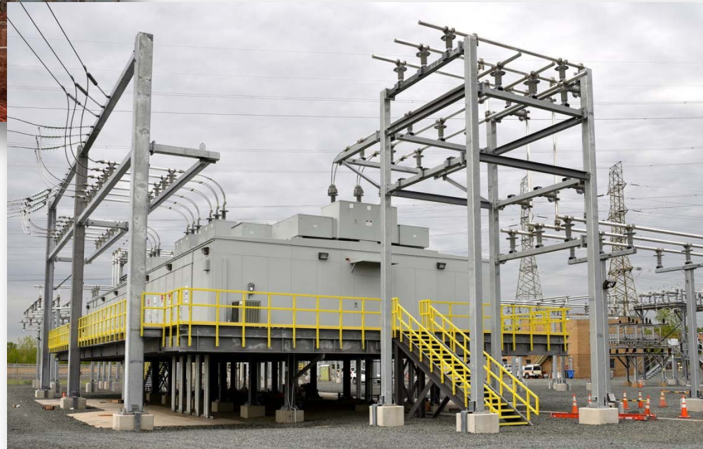
Sewaren Switching Station – After
